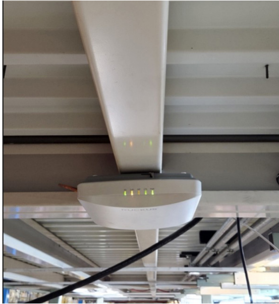
AP mounted under work platform
